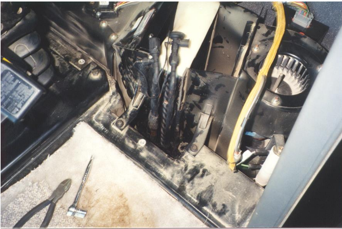
Evaporator in place alongside heater assembly.
